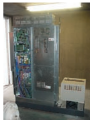
Elevator Control Board Refurbishment CV260RN
