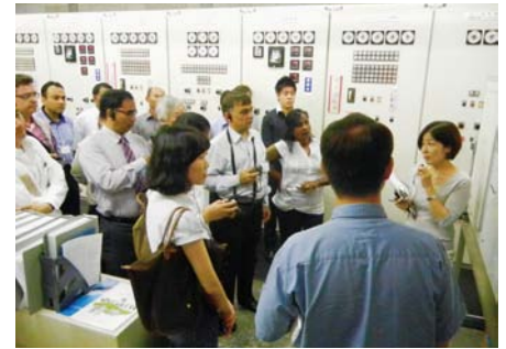
Participants touring the power generation facility/ integrated energy management system of Hotel New Otani.
