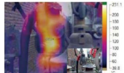
Figure 2. IR thermographic identification of a loose transformer connection. The inset is a view of the entire device.
