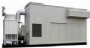
Cogeneration system at Sendai Nikon Corporation
